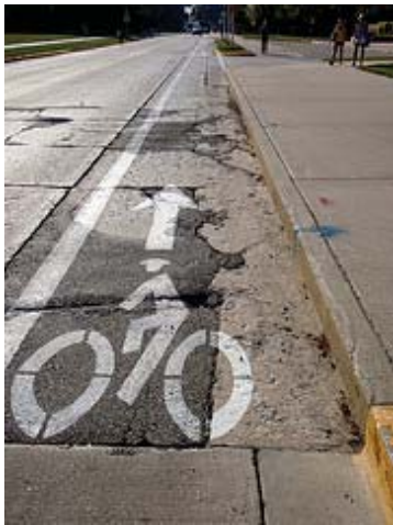
Urbana - crumbling bike lane
