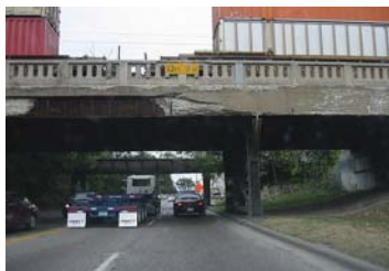
Stickney - crumbling viaduct
